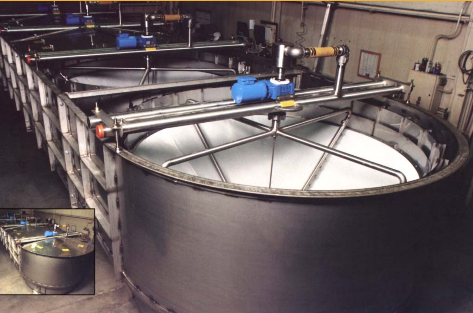
Fig. 3: A Multipack modular unit using four Fiber Retriever modules. Insert photo shows covers in place.
